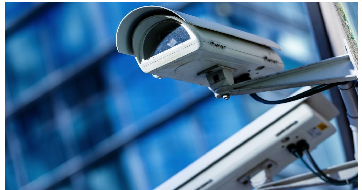
CCTV CAMERA SURVEILLANCE
